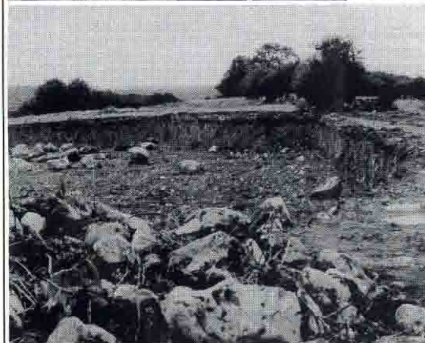
The new clubhouse will be erected in the excavated area overlooking the 18th green at Castlequarter.
