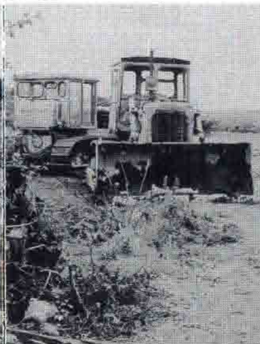
Some of the machinery used in the construction of Gort's new 18 hole golf course.
