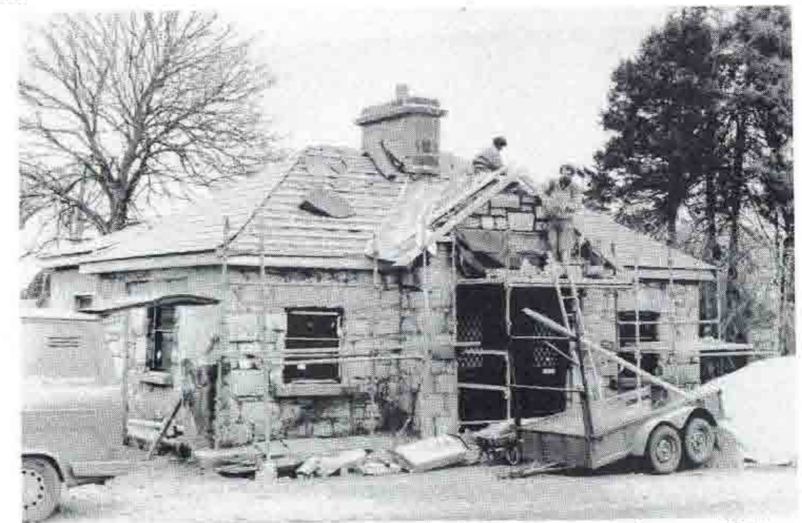
Restoration work in progress on the Gate Lodge in Coole last February. The lodge, now the property of Robin Marcus of Lough Cutra is being tactfully restored inside and out. Full marks to Mr. Marcus for a job well done.
