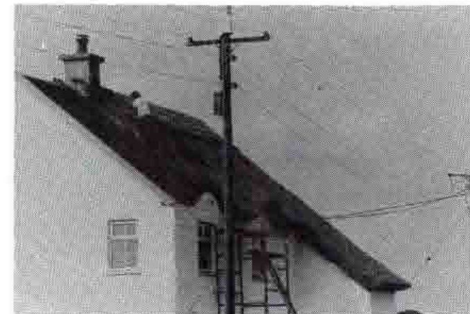
A rare sight in Gort! A thatcher at work on the Galway Road last Autumn.
