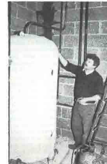
Séamus Glynn at work on the heating system for Gort Community Centre.
