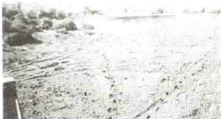
Work continues on Gort's new dump. When completed it will be one of the most modern dumping sites in the West of Ireland.
